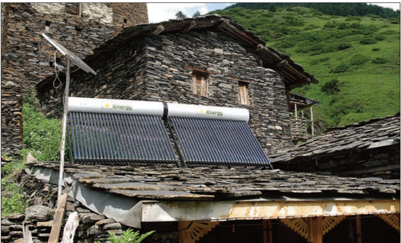
Solar panels installed by the Czech Development Agency in Tusheti
